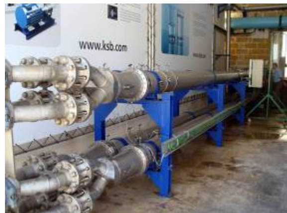
Fig 11 – SALTEC rack on a 4.50 MLD line (Abandoned equipment)
