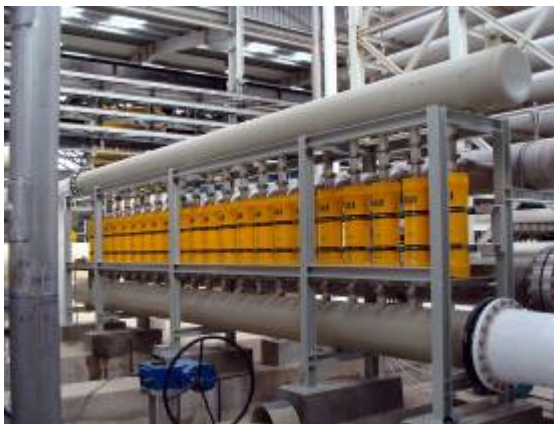
Fig 8 – PX rack on a 20 MLD line
