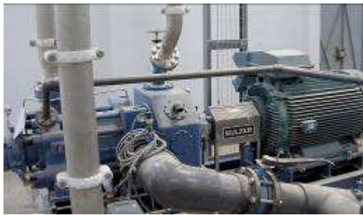
Fig.3 - HP pump with Pelton turbine
